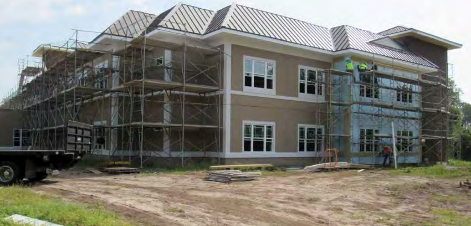
Construction of the new and expanded Health, Rehabilitation and Memory Care Center
